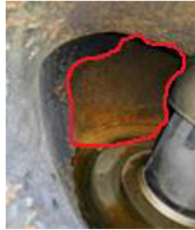
Fig. 4. The erosion damage morphology of upstream body of black water angle valve LV-0301A.
